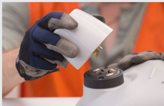
Figure 34 – A smart sensor light point controller plugs in to a luminaire mounted NEMA receptacle (Philips)
