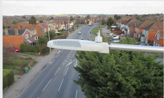
Figure 19 – Individually controlled and metered LED luminaire in UK (Telensa)
