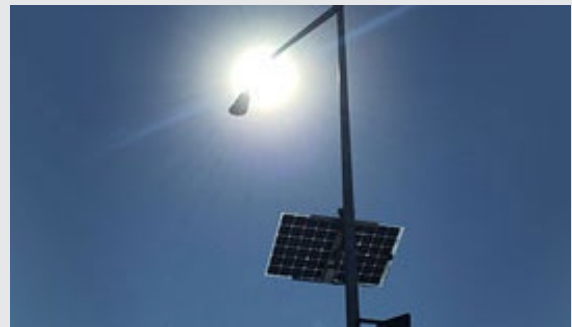
Figure 27 – Solar PV on-grid column (Petra Systems)
